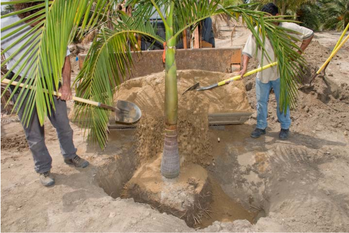
Figure 2. The palms were replanted using builder's sand, as here with king palm, or native site soil as the backfill medium (Photo © Copyright 2008 by D. R. Hodel).
