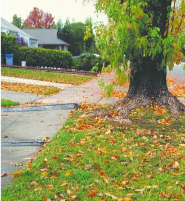
Sidewalk upheaval adjacent to a wide planting strip, due to shallow tree roots. (Fig. 2)
