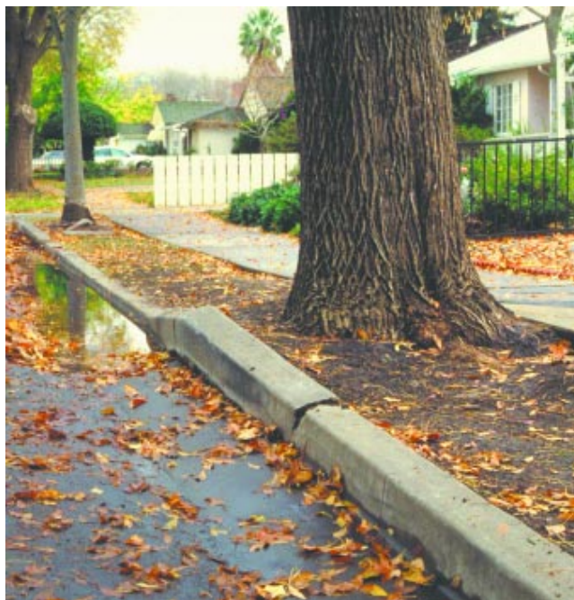
Severe sidewalk and curb damage due to shallow tree roots and narrow planting strip. (Fig. 1)
