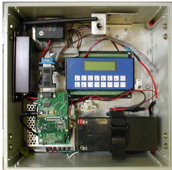
Figure 4. Field controller with embedded controller and wireless module (base node).
